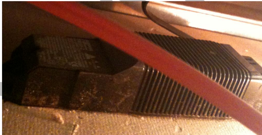
Figure 6 - magnetic transformer in situ in ceiling space
